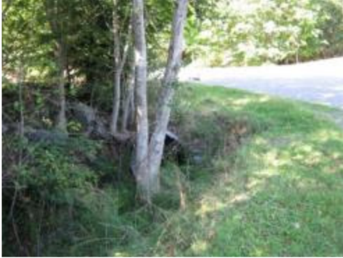
Enos Creek (S1) at Swallow Rd and Dolphin Drive looking upstream at 1,500 mm dia
