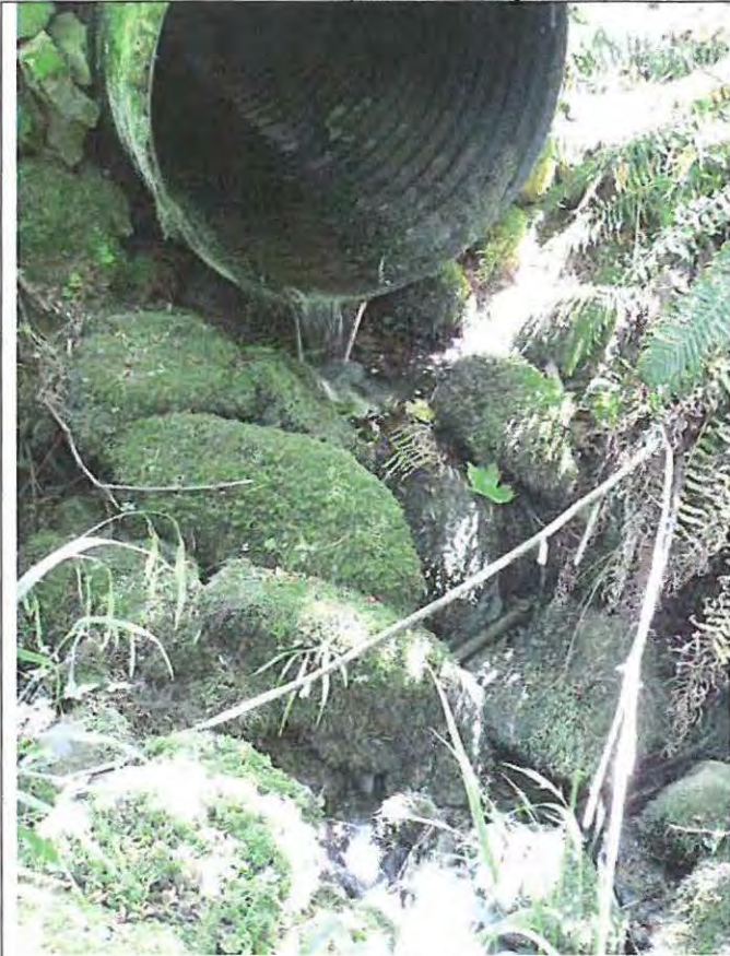
Photograph 4. June 2014. View of the outlet of the culvert at Taylor Bay Road.
