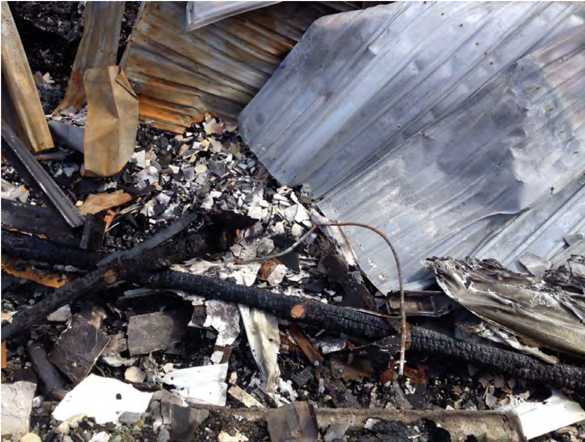
After Fire Damage
