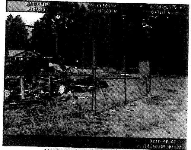
Unsecure Construction Fence
