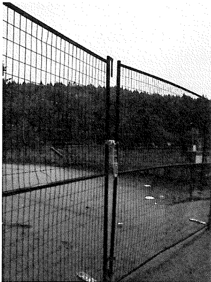
Unsecure Construction Fence
