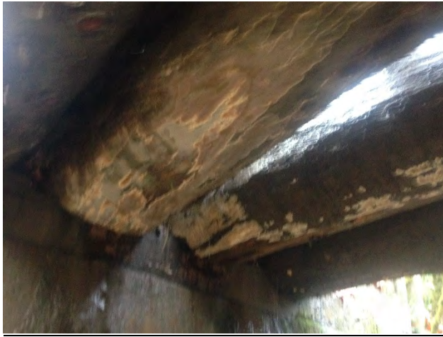
Underside of Log Stringers – note presence of biological growth
