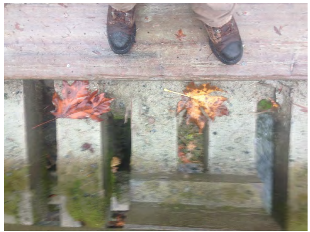
Muddy debris on Deck
