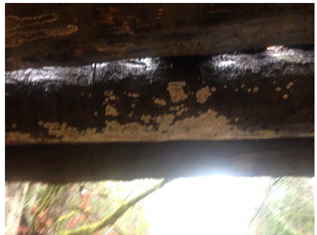
Underside of Log Stringers – note presence of biological growth
