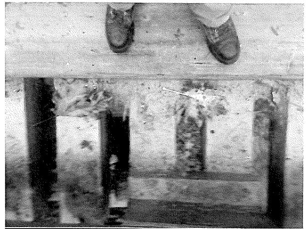
Muddy debris on Deck
