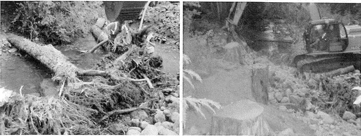
Anchoring of imported large woody debris instream, rootwads placed along bank, bank resloped with native alluvium and revegetation by seeding, bioengineering and native plantings.
