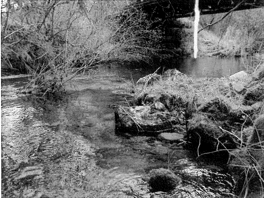
Downstream angled view along right bank abutment riprap upstream of the bridge. Note flow is deflecting off the tip of riprap and other fill that juts into the channel. This is deflecting flows toward the left bank and left bridge abutment and may be contributing to small and localized erosion.
