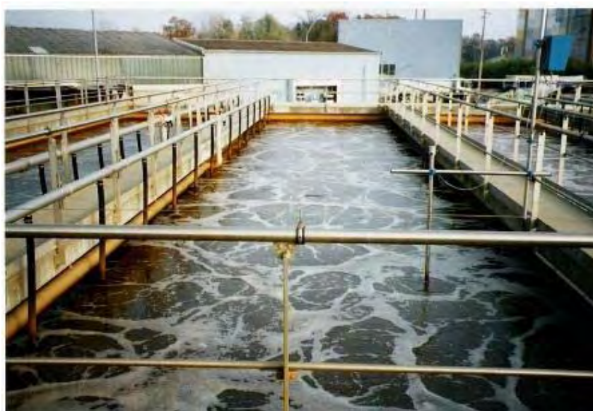
Figure 1 An Activated Sludge Aeration Tank
