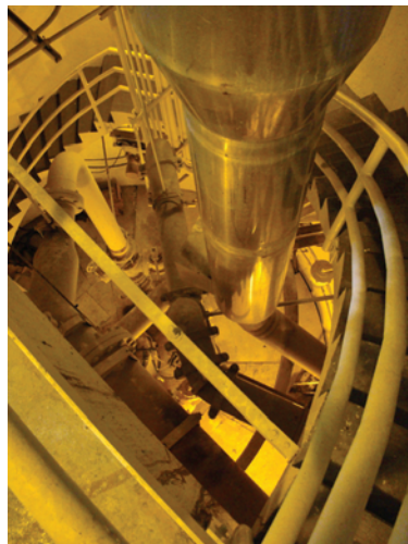
VIEW FROM INSIDE THE CHASE RIVER PUMP STATION
