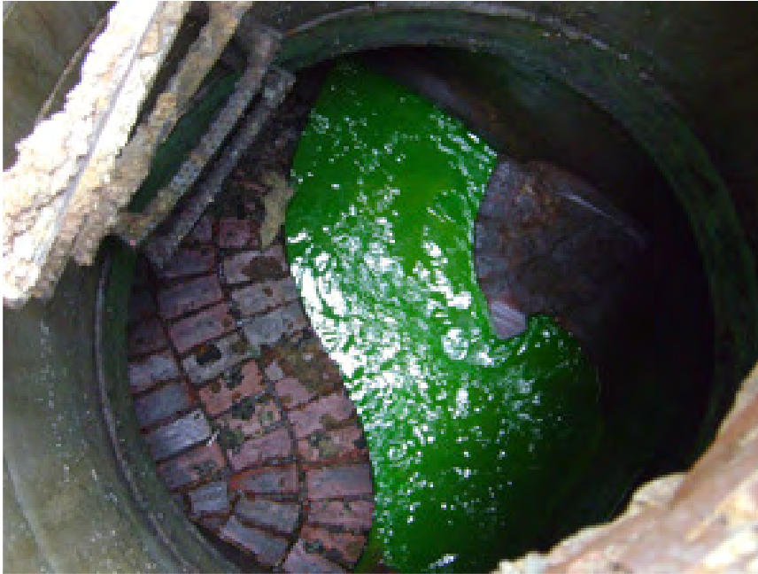
Figure 7. Dye is observed in a manhole downstream of an inflow source
