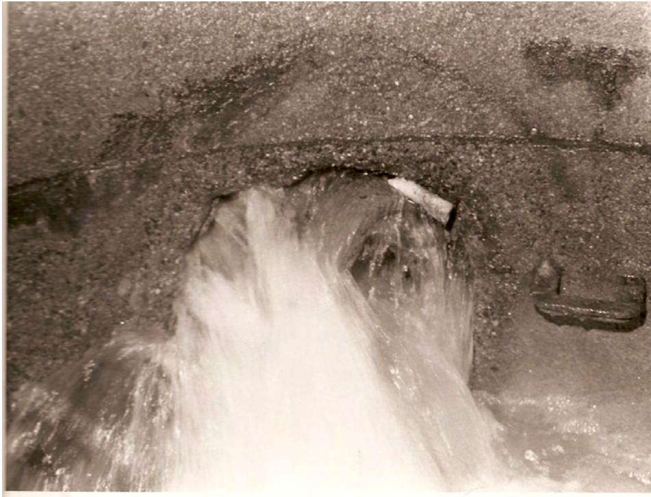
Figure 12. Significant infiltration of water into a damaged manhole.
