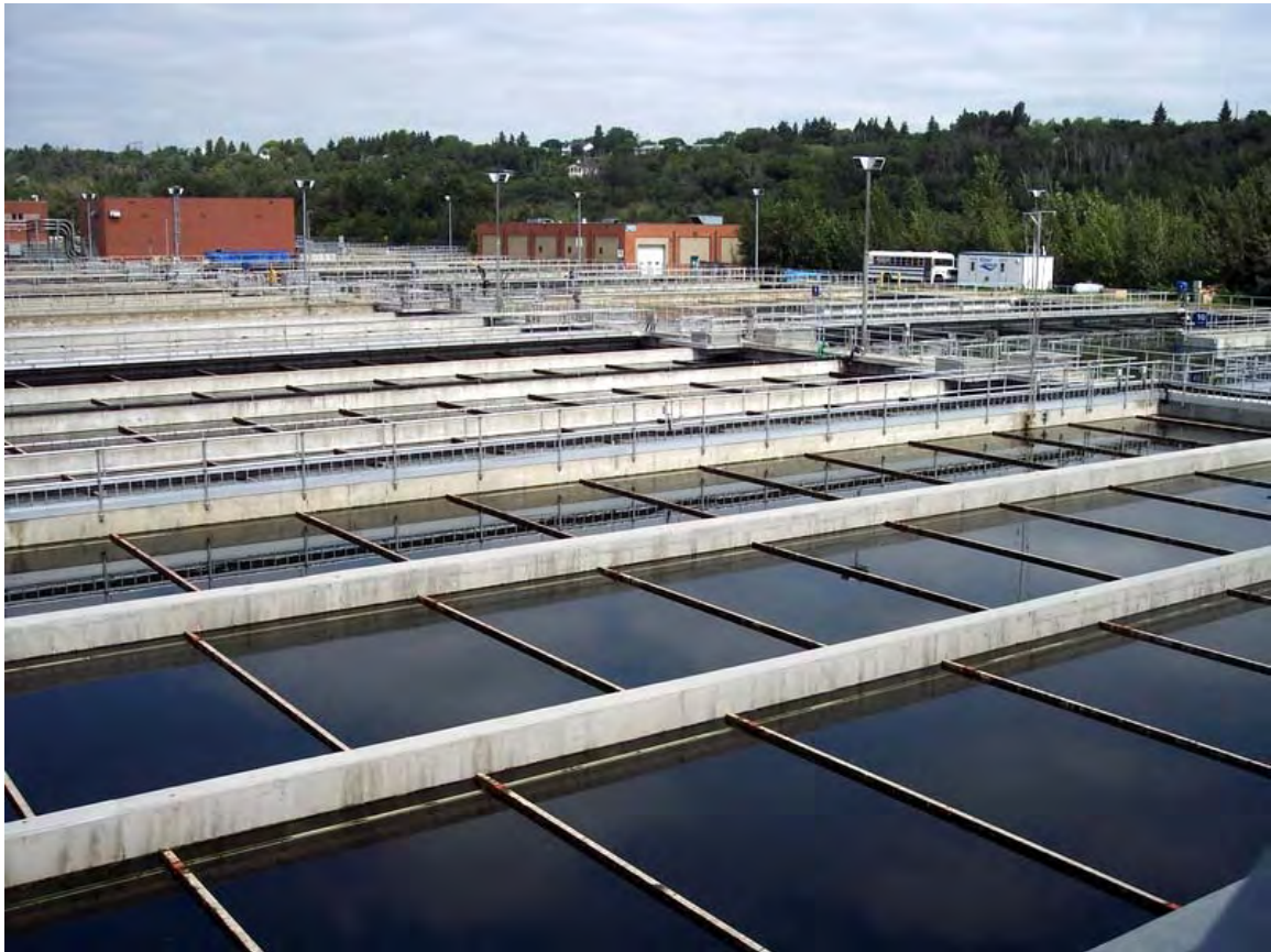
Figure 9 City of Edmonton Rectangular Secondary Clarifiers
