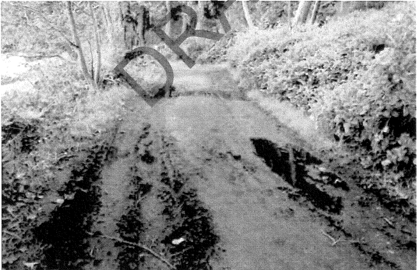
Figure 14. Main park trail showing rutting and mud
