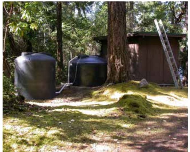
Two poly tanks storing water from a small pump house building.
