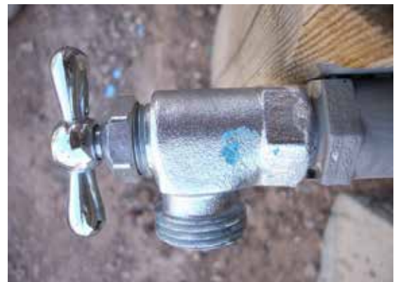
Hose bib containing non-potable water must be labelled clearly.
