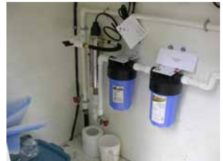
Smaller capacity sediment filters and UV light.
