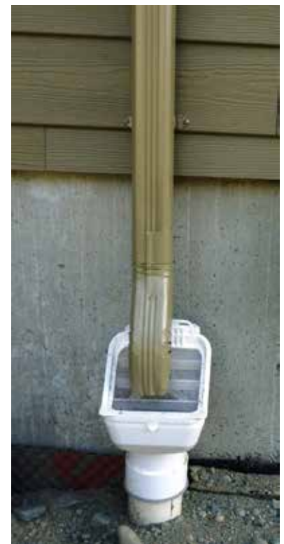
Self cleaning leaf trap between downspout and underground transport piping.
