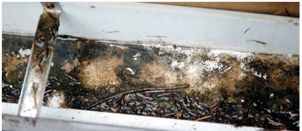
Spring pollen and debris in open gutter.
