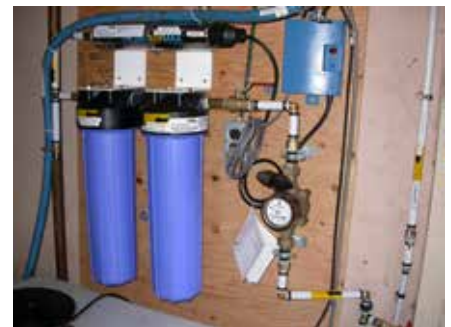
Dual-particle filters and U.V. light with water metre.
