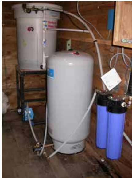
Biosand jet pump pressure tank and particle filters.
