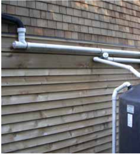
Downspouts to catchment pipe and into tank.
