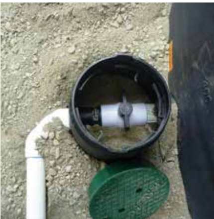
Two-inch tank exit valve.
