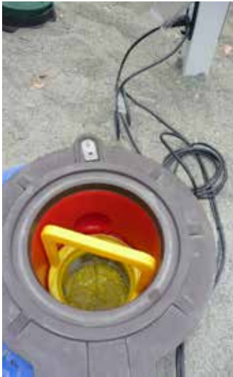
Water flowing into filter basket of whole house; combined filter and pump chamber.
