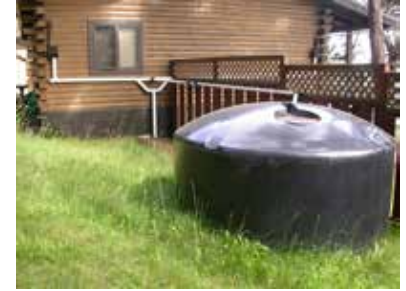
Wall-mounted pipe to 1660 gallon tank.
