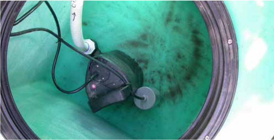
Simple pond pump in transfer tank.
