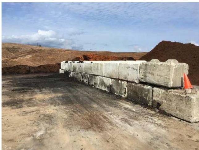
Photo: Lock blocks set up on the hog fuel pad at Harmac for biosolids stockpiling and soil mixing operations. Photo credit SYLVIS Environmental
