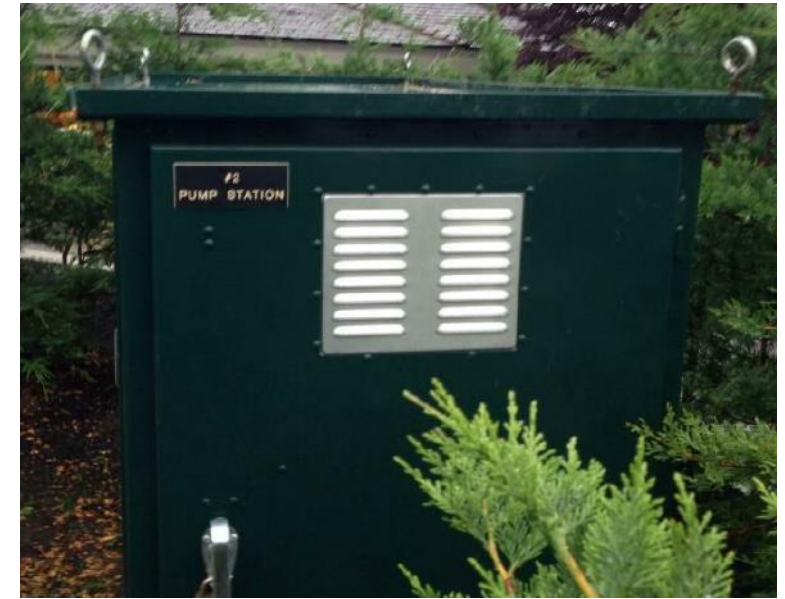
Nanoose Pump Station #2 Electric Kiosk
