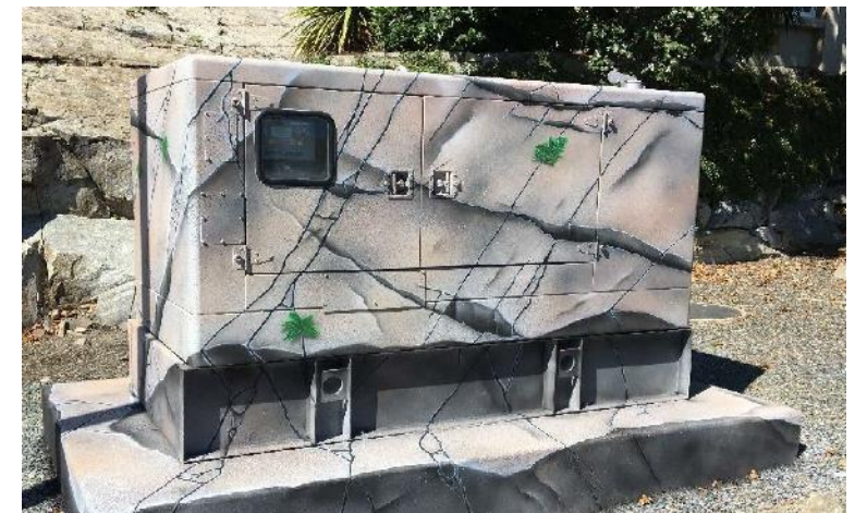
Nanoose Pump Station #2 Generator
