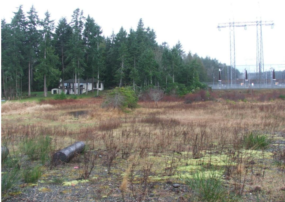
BC Hydro Substation and Power Cables (Looking Inland from Shoreline)
