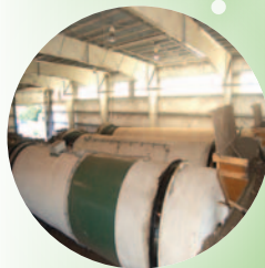
The composting process starts in a rotating composter drum.
