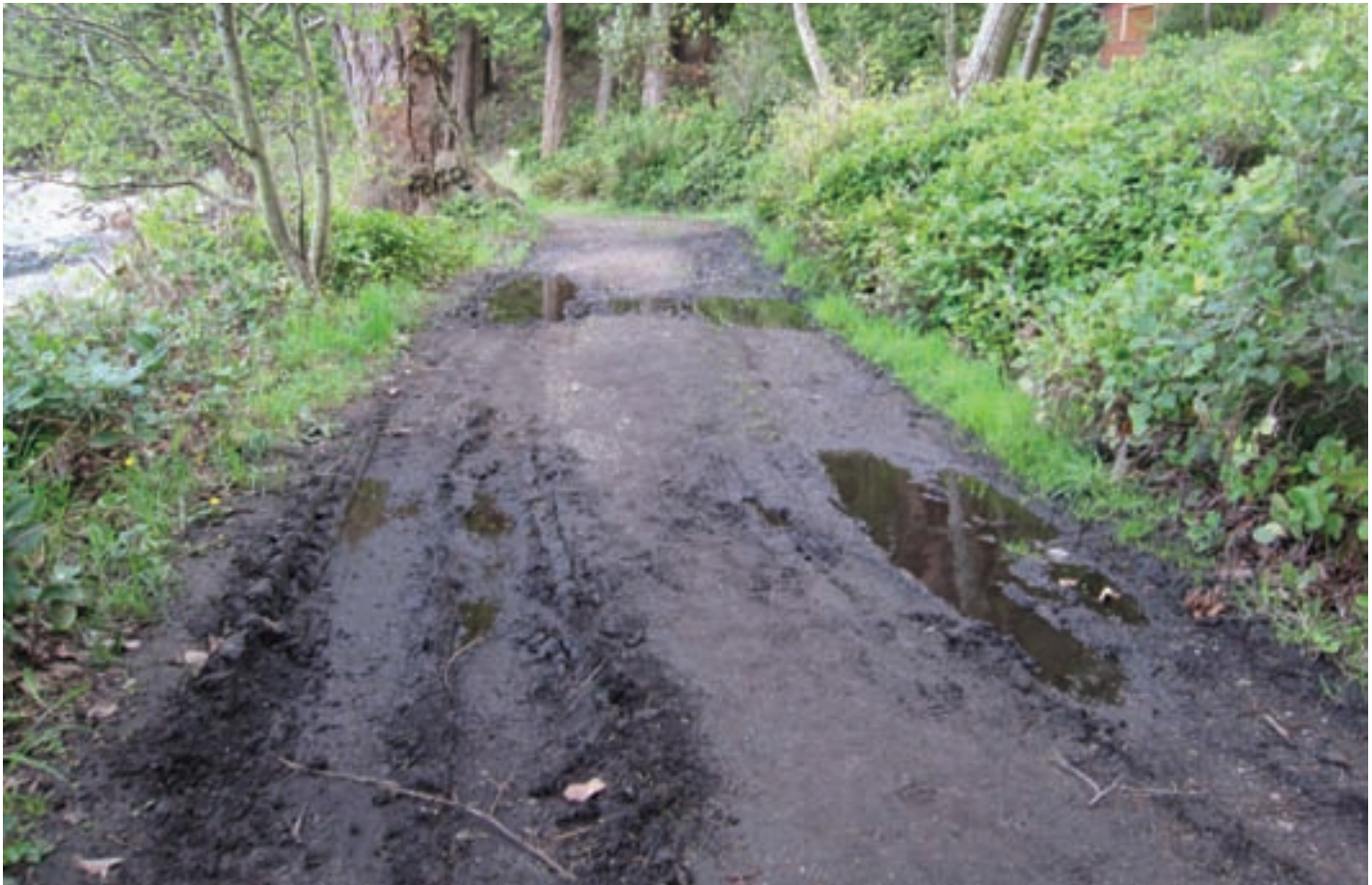
Figure 14. Main park trail showing rutting and mud
