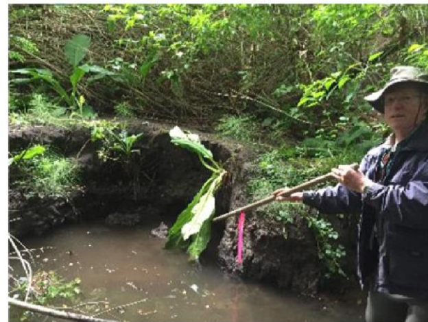
Metral M1- erosion from storm water
