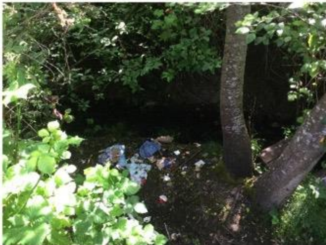
Photo 3) R2, 5th Street culvert garbage and drug debris
