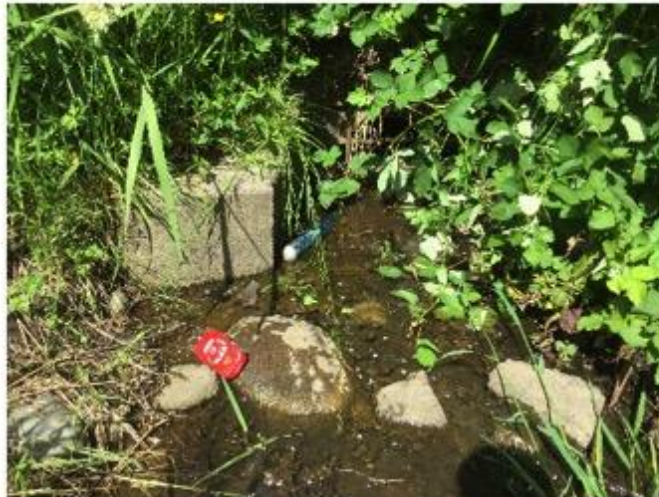
Photo 2) Pine street culvert effluent contributing poor quality water and sediments
