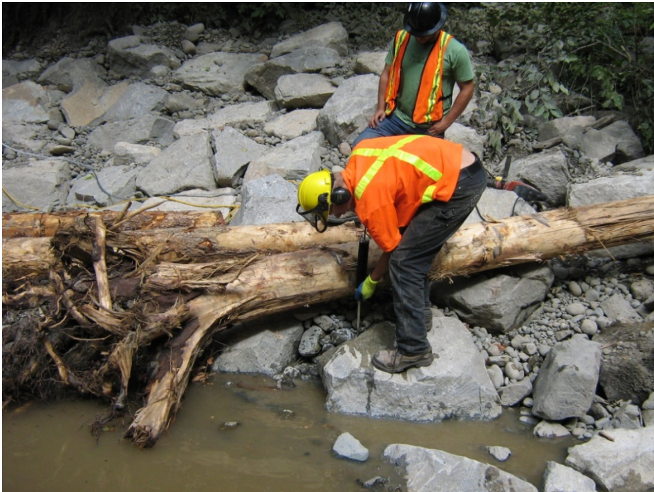
Photo 9. The BCCF crew anchored the LWD to boulders using wire rope, clamps, and epoxy.
