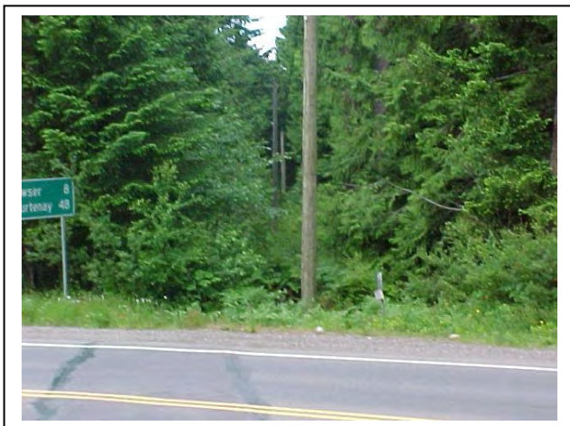
Hydro power line on R/W, highway view
