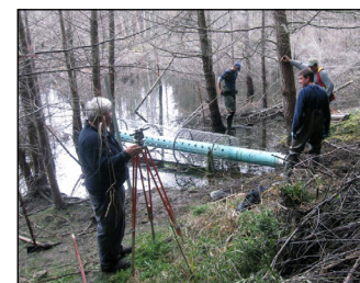
Installation of Clemson Pond Leveller in October 2009 by RDN and TNT staff (RDN photo)
