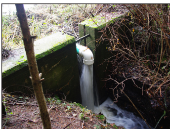
Concrete weir and pond leveler controlling water levels at the outflow of the wetland area on the west boundary of the Coats Marsh RP. (FBER Ltd photo)
