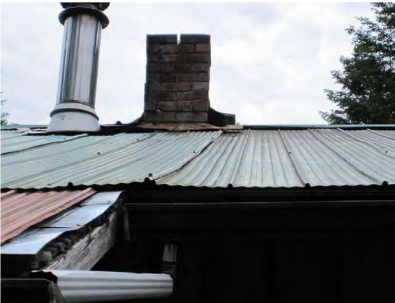
Roof and brick Chimney are in poor condition.
