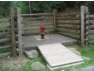
Photo. Fire hydrant near ferry terminal.
