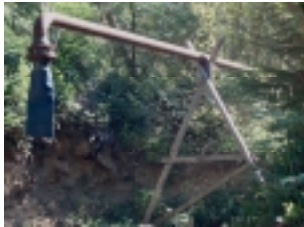
Photo 23. Tanker refilling site at Crosley Road: a gravity-operated pipe is connected to a former CPRail 15,000 gallon tank car.
