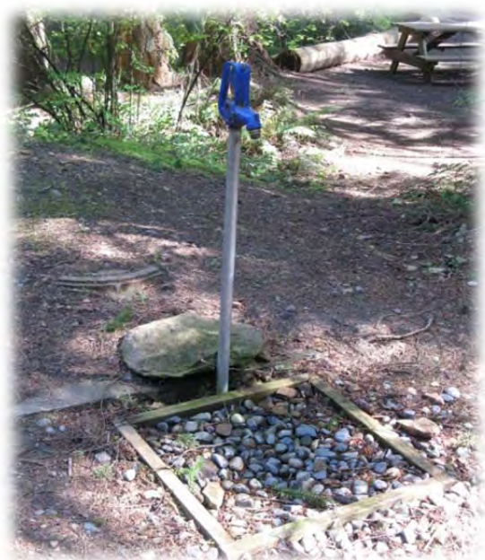
Standpipe for water supply in Descanso Bay Regional Park
